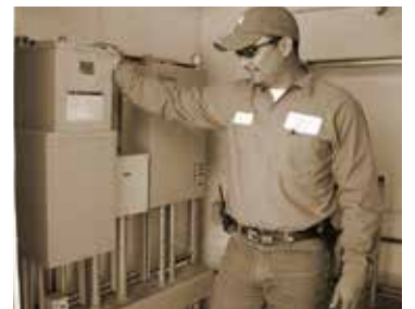
2012 The City of Bovina wrapped up a CDBG project to rehab water wells and install water meters throughout the city, as well as provide a generator to pump.
